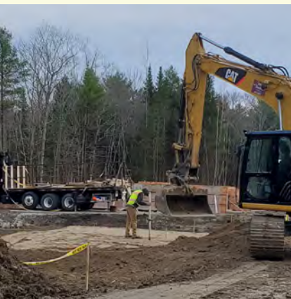
Foundations are being poured on Jasper Drive for custom homes and Quarry Cottages.
