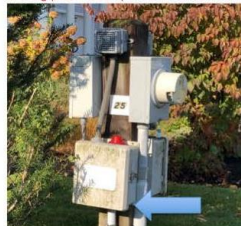
1. Pump Panel Control Box
