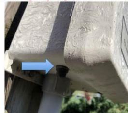
2. Alarm Shut-off Button
