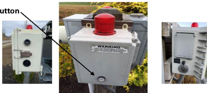
Warning: please do not open the control box to shut off the alarm – high voltage wiring inside
